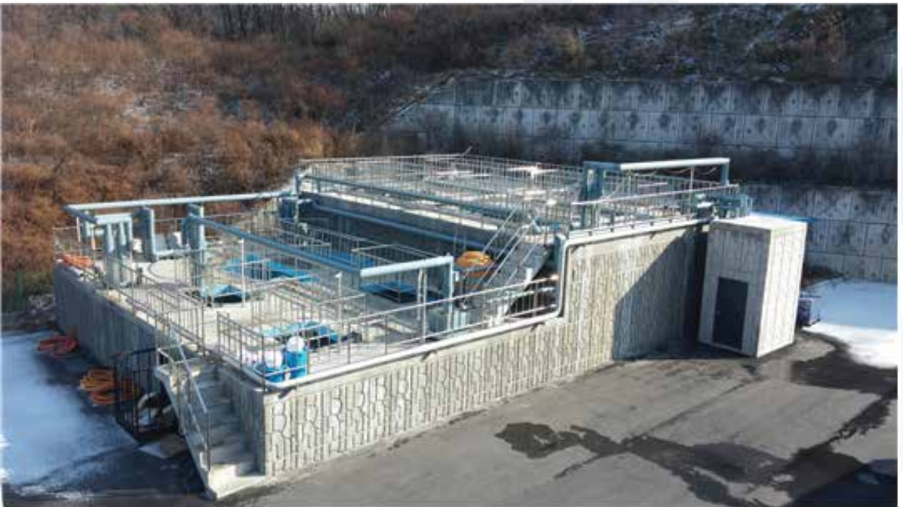
DMF (Dimethylformamide) Wastewater treatment plant
